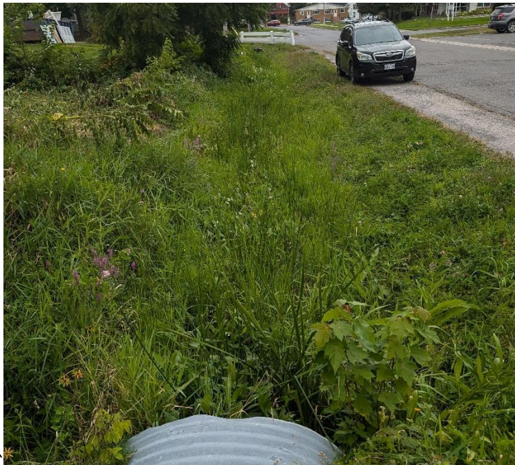
Figure 18: Looking downstream from the culvert on the Main Drain between Victoria and Caleb Street at Station \pm 10+54 .
