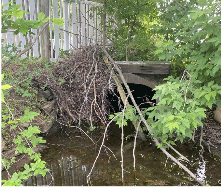
Figure 7: Showing the downstream end of the enclosure at station \pm 5+52 traveling underneath Fred Street. The enclosure at this end appears to be constructed from a repurposed steel oil tank.
