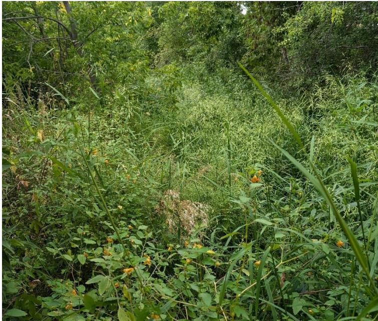
Figure 10: Significant vegetation growth at station ±6+54.
