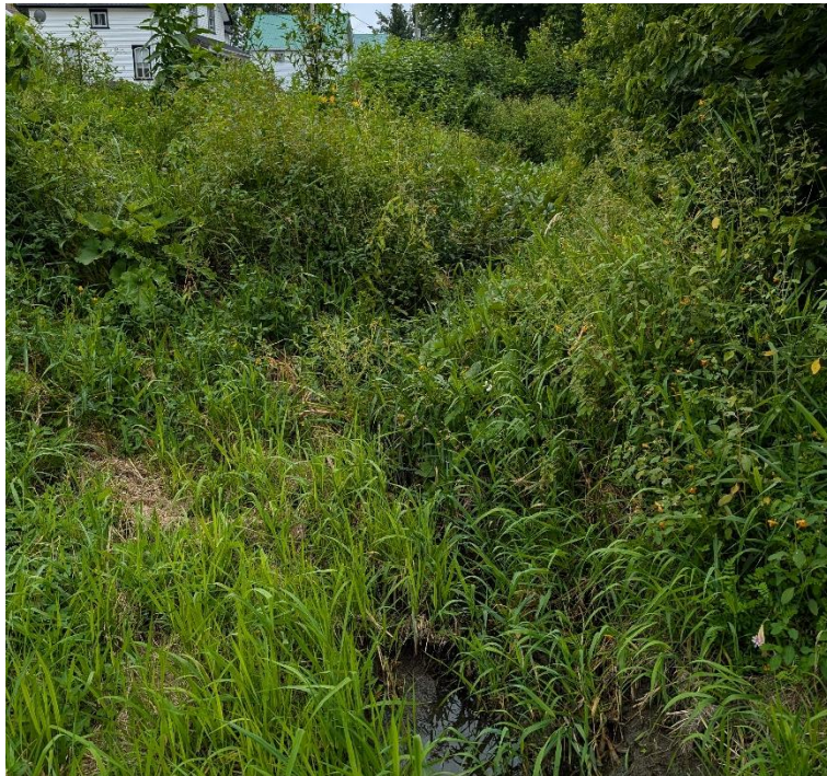
Figure 22: Looking upstream front inlet of culvert crossing Ottawa Street. Significant vegetation growth was observed in this segment. Photo at station \pm 14+40 .
