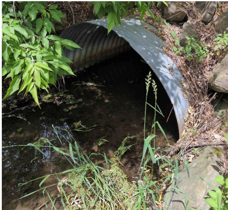
Figure 4: Upstream end of the enclosure at station \pm 3+97 running beneath County Road 38. The opening measured 78".
