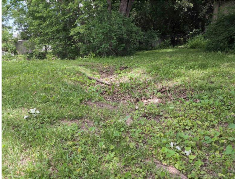
Figure 5: Showing a depression in the ground at station \pm 4+26 above the enclosure which crosses County Road 38 suggesting a possible failure.
