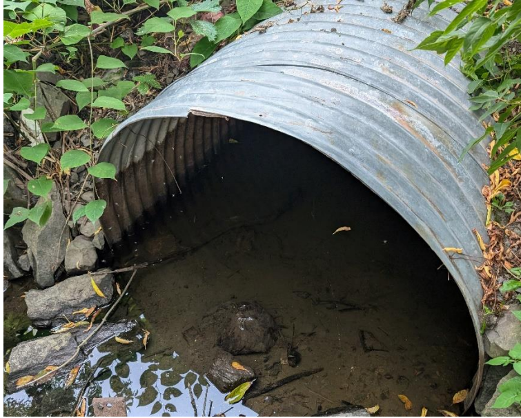
Figure 9: Showing the downstream end of the enclosure at station 6+42 which crosses May Street. The opening of the CSP was measured at approximately 60”.
