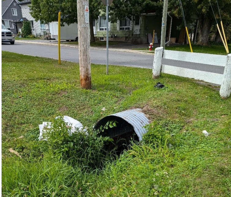
Figure 19: Photo at station \pm 10+90 : Showing inlet of the 600' enclosure on the Main Drain that terminates at station \pm 12+82 , just north of Main Street. The opening measured approximately 60" across.
