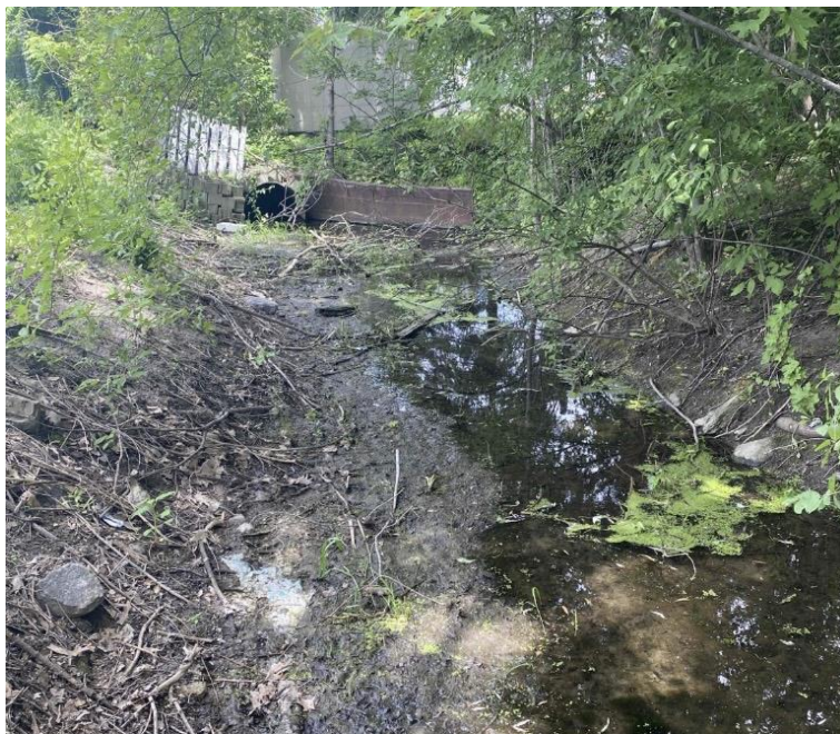
Figure 6: Showing the section of drain between stations \pm 4+30 and \pm 4+59 . At the far end exists the upstream end of the enclosure that crosses Fred Street. The section of pipe visible at the inlet is CSP.
