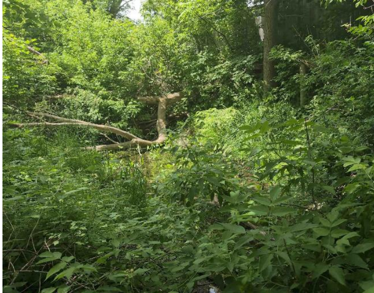
Figure 27: Example of fallen trees and debris in the Diversion Drain behind the homes on Victoria Street
