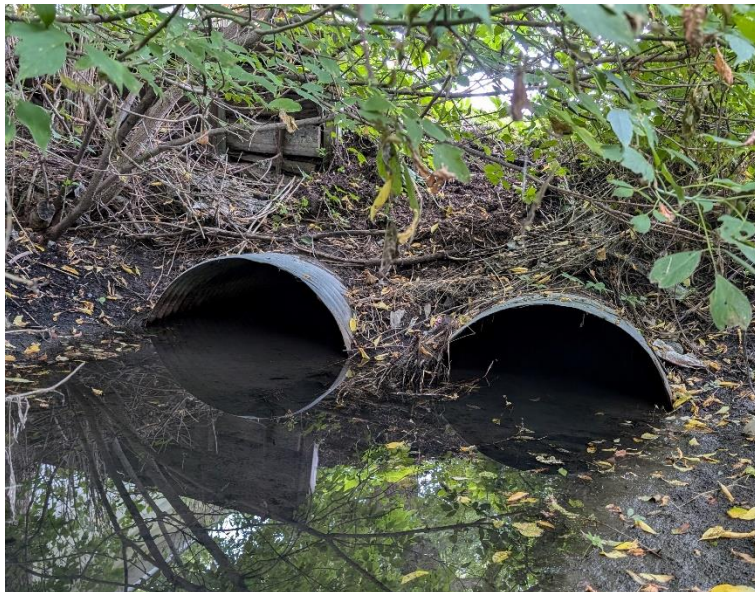
Figure 20: Showing the downstream end of the Main Drain enclosure which crosses Main Street. Both pipe ends are CSP and measured approximately 39" across their openings. Pipes appeared to be over 50% full of sediment. Photo taken at Station \pm 12+82 .
