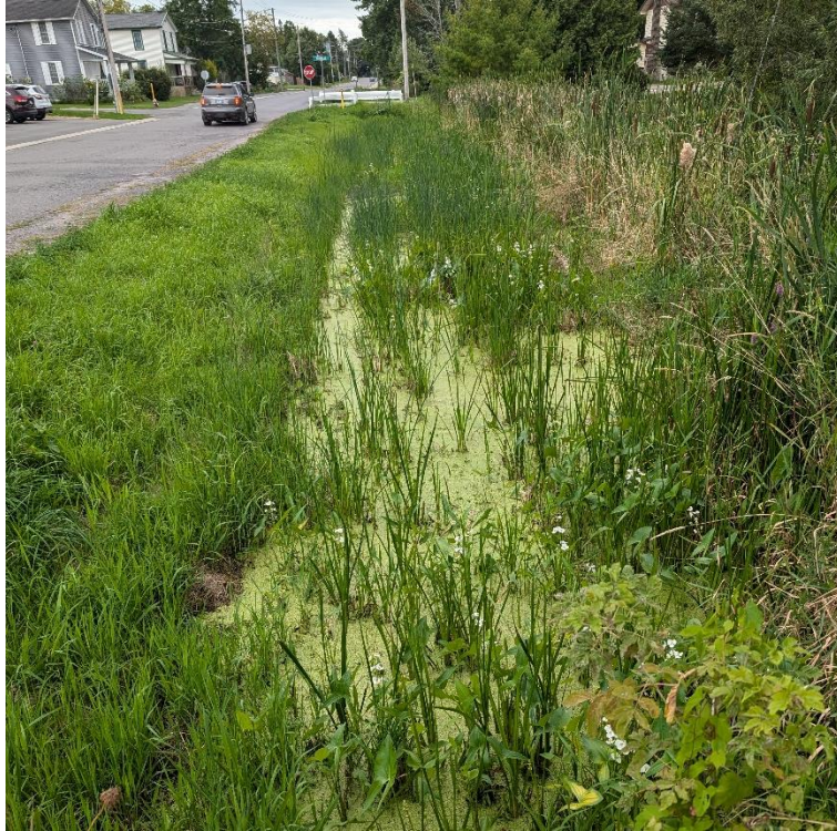
Figure 17: Looking upstream from the culvert on the Main Drain between Victoria and Caleb Street at station \pm 10+50 .
