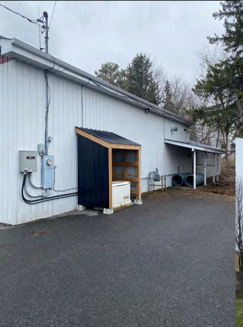
North Side of station with stand-by generator and office exit,
