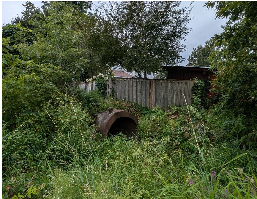
Figure 12: Downstream end of the enclosure crossing York Street at station \pm 7+68 . Constructed from non-standard repurposed steel pipe/oil drum.
