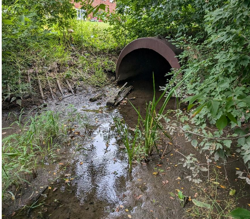
Figure 11: Upstream end of the enclosure at station \pm 6+92 that crosses under York Street. Constructed from non-standard repurposed steel pipe/oil drum.
