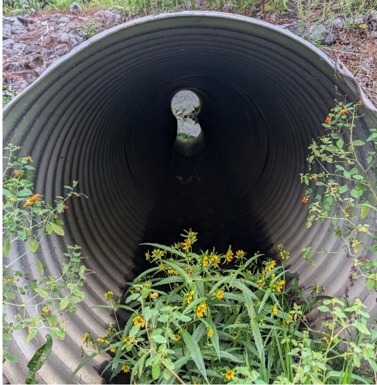
Figure 23: CSP culvert crossing Ottawa Street on Main Drain. Measured approximately 60" across. Photo at station ±14+60.
