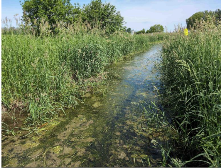
Figure 29: Section of the drain at station ±41+52 where it appears recent maintenance has been completed.
