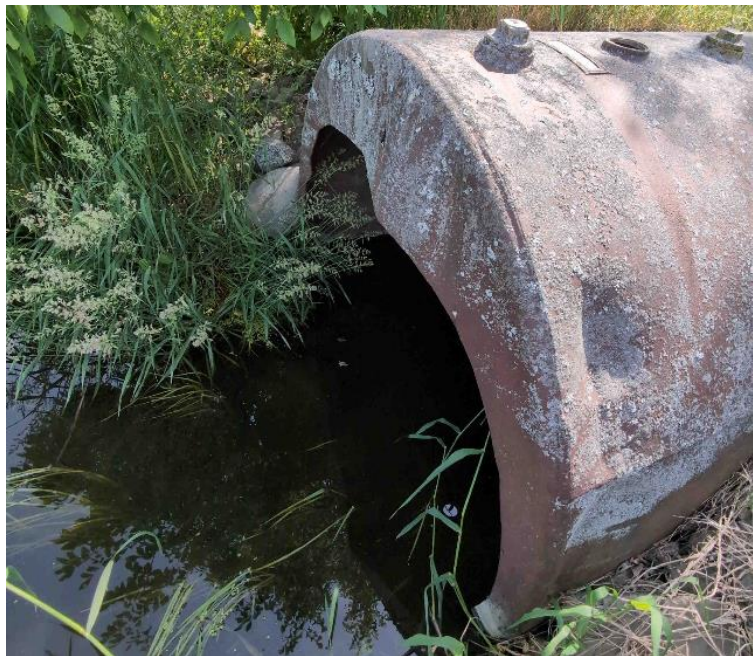
Figure 30: Showing an example of a culvert suspected to be made of repurposed, steel oil drum at Station ±42+51.
