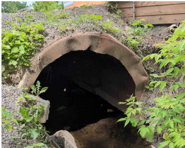
Figure 8: Showing the upstream end of the enclosure at station \pm 5+87 which crosses May Street. This end of the enclosure is presumably constructed from a repurposed steel oil tank.
