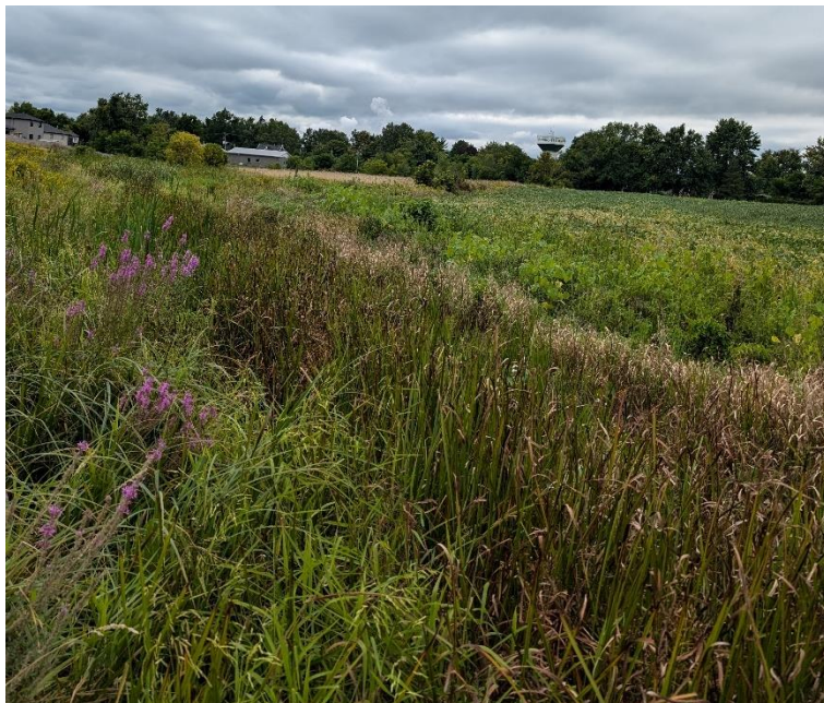
Figure 24: Showing significant vegetation growth in the section of the Main Drain north of Arora Crescent at station ± 18+57.
